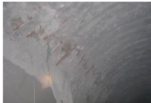
Figure 2 Concrete has fallen off
