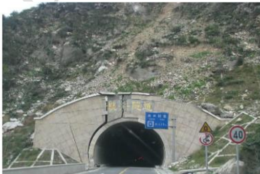
Figure 1 Cracks at the entrance
